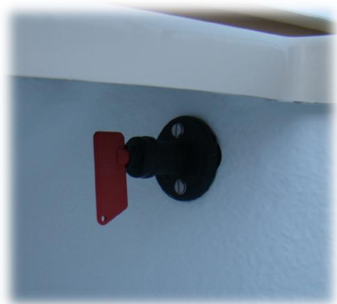
* main power switch
